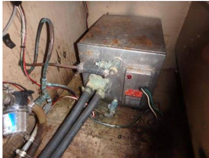
Hot water heater is old and replacement should be considered. Water heater AC wiring is not compliant.
